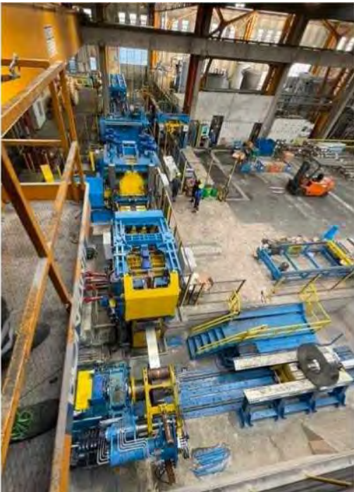
Civate plant - Levelling and blanking system with automatic packaging
